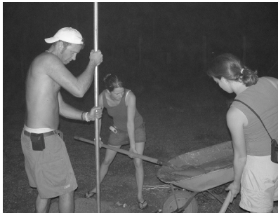
Daren Beaupre (bioengineer), Maureen Wrobel (OR nurse), and Sarah Syndacker mixing cement to anchor a pole for a volleyball net at the orphanage
